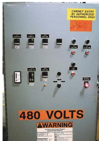
Fig.5.9 Written and warning instruction on the control panel
