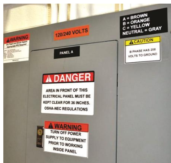
Fig.5.10 Written and warning instruction on the control panel
