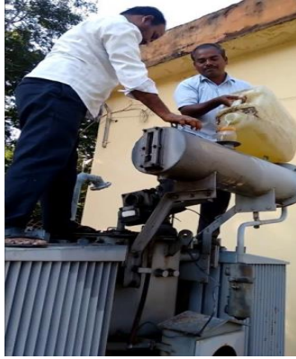
Fig.5.21 Manual filling of oil in the transformer
