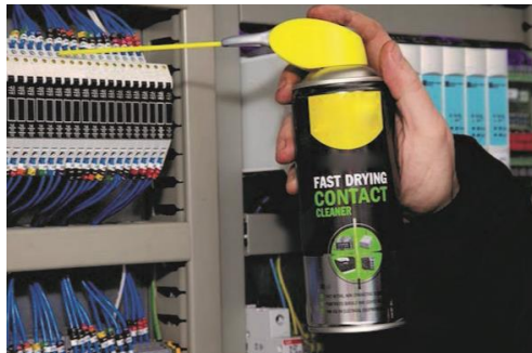
Fig.5.7 Equipment cleaning spray
